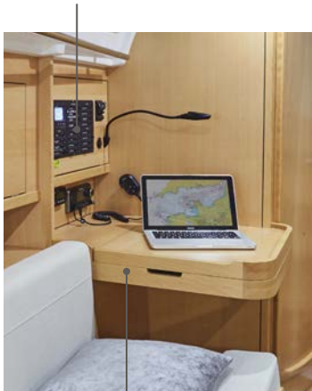
A clear and accessible electrical panel
