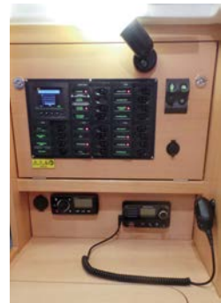
Full featured electrical panel
