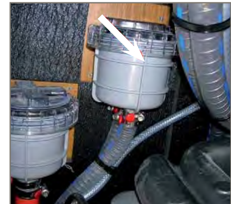
WATER FILTER OF THE GENERATOR
