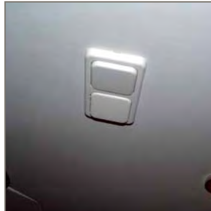
LIGHTING SWITCHES DIRECT - SALOON
