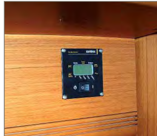
SHORE POWER SOCKET / GENERATOR INVERTER SWITCH
