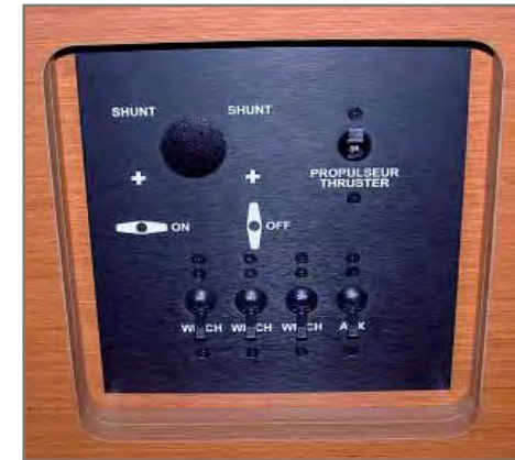
AUTOMATIC BREAKER PANEL
