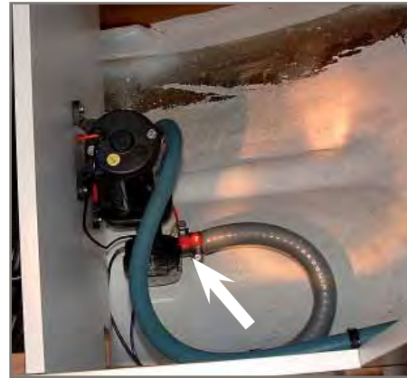
SUPPLY VALVE OF THE DECKWASH PUMP
