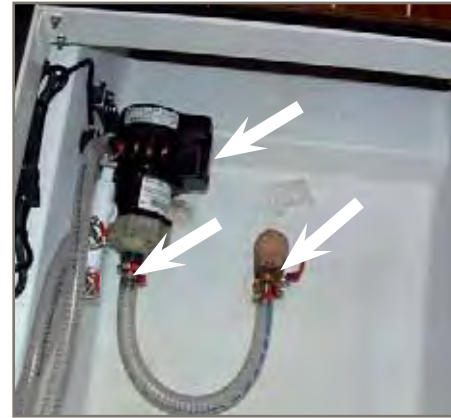
PUMP + SUPPLY VALVES + FILTERS
