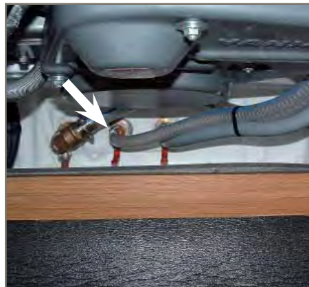
WATER INLET VALVE OF THE GENERATOR
