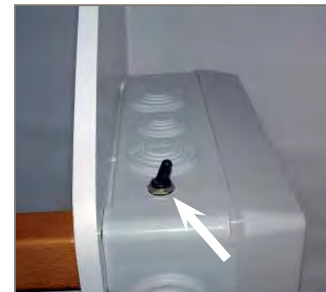
DECKWASH PUMP SWITCH
