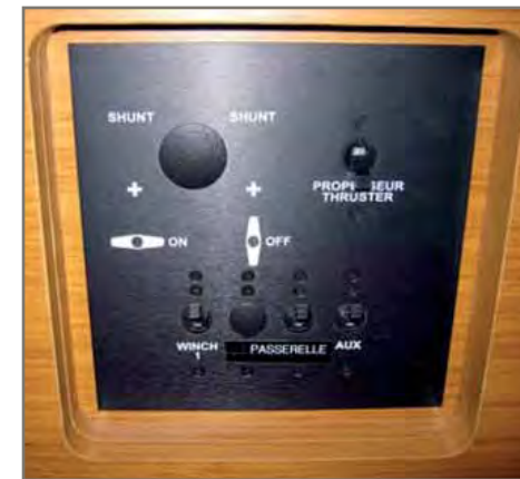
AUTOMATIC BREAKER PANEL
