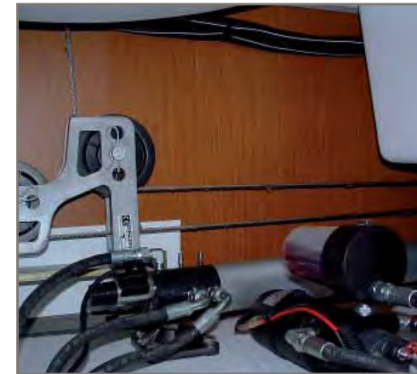
ACCESS TO THE STEERING CABLES AND TO THE AUTOPILOT RAM
