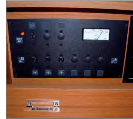
AUTOMATIC BREAKERS OF PUMPS + AIR CONDITIONING UNITS
