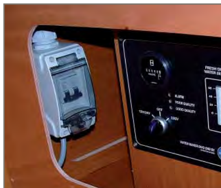
WATERMAKER AUTOMATIC BREAKER
