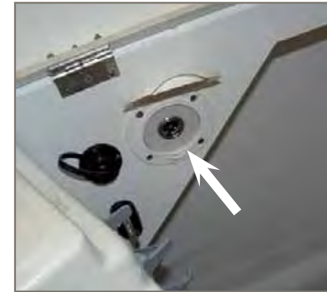
WATER INLET DECKWASH PUMP
