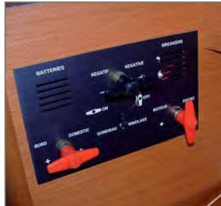
CUTOUPS + AUTOMATIC BREAKERS PORT AFT CABIN
