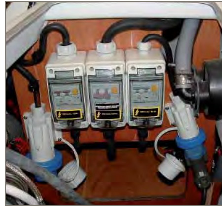
SHORE POWER SOCKETS + AUTOMATIC BREAKERS
