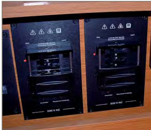
SELECTORS SHORE POWER SOCKETS / GENERATOR
