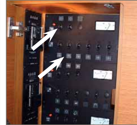
AUTOMATIC BREAKERS OF PUMPS + AIR CONDITIONING UNITS
