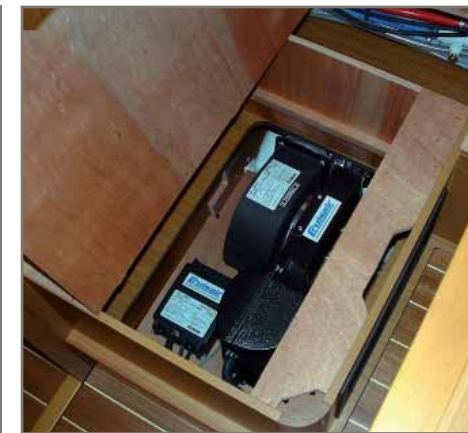
AIR CONDITIONING UNIT
