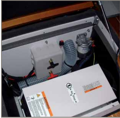
GENERATOR + CUTOUTS + FUEL OIL FILTER
