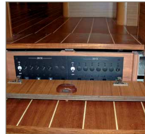
AUTOMATIC BREAKER PANEL
