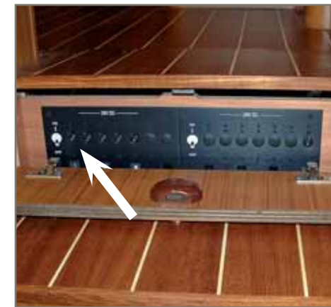
AUTOMATIC BREAKER OF THE ELECTRIC WINDLASS
