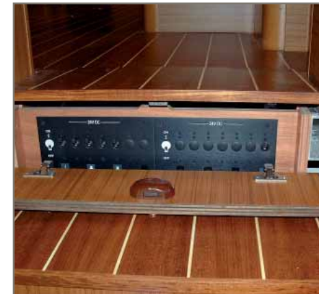
AUTOMATIC BREAKER PANEL
