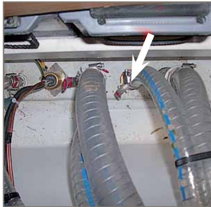
WATER INLET VALVE OF THE GENERATOR
