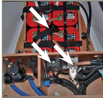
BATTERIES + FUSE + AUTOMATIC BREAKER
