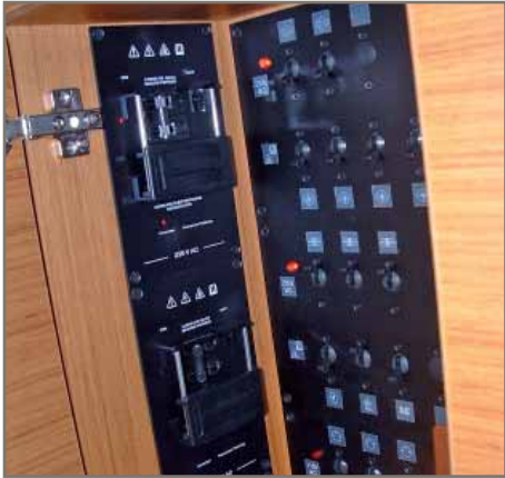
230V ELECTRICAL PANEL + SELECTION PANEL
