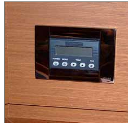
AIR CONDITIONING CONTROL
