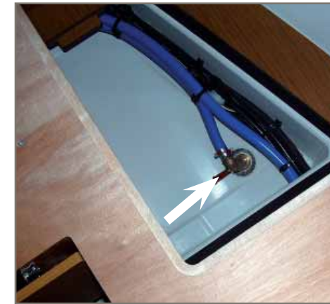
SUPPLY VALVE OF THE DECKWASH PUMP
