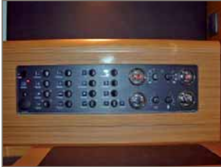
ELECTRICAL PANEL OF CHART TABLE
