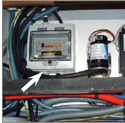
GENERATOR AUTOMATIC BREAKERS
