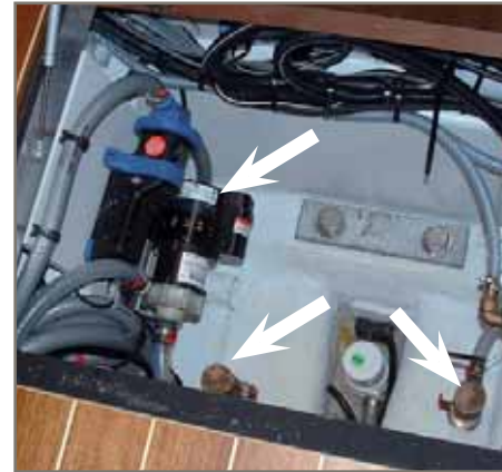
PUMP + SUPPLY VALVES + FILTERS
