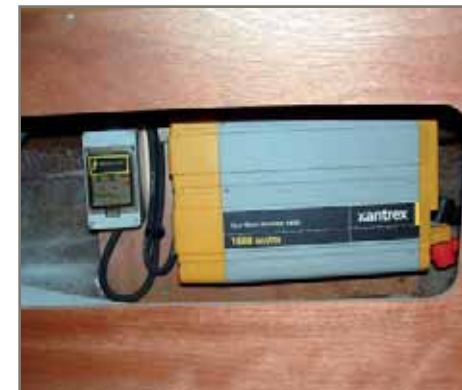
INVERTER + AUTOMATIC BREAKERS
