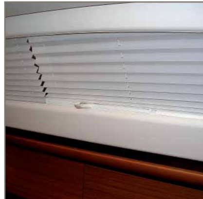
BLIND - SIDE DECK WINDOW
