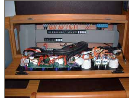
AUTOMATIC BREAKERS BEHIND THE ELECTRICAL PANEL
