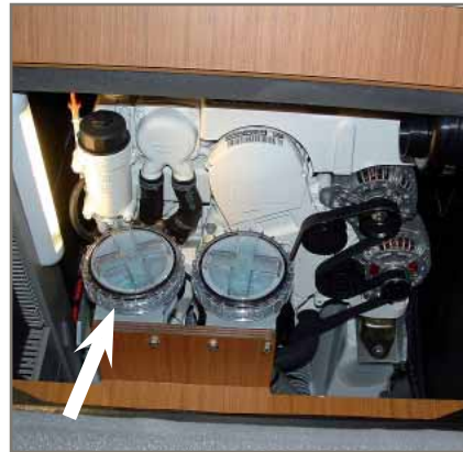
WATER FILTER OF THE GENERATOR
