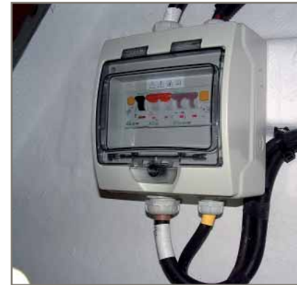
AUTOMATIC BREAKERS OF THE SHORE POWER SOCKETS
