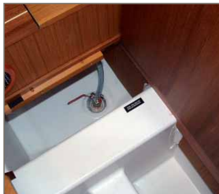
SEA WATER SUPPLY VALVE
