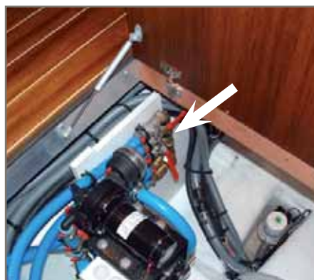
VALVES TO SELECT THE TANKS
