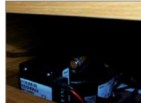
24V ENGINE OF THE GALLEY REFRIGERATOR
