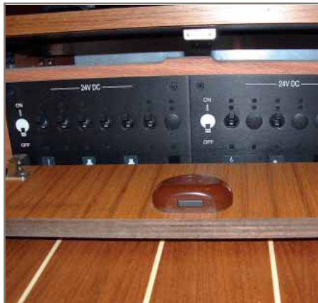
ELECTRICAL PANEL UNDER SALOON STEP
