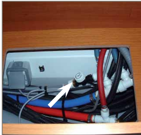
WASHING MACHINE SUPPLY VALVE
